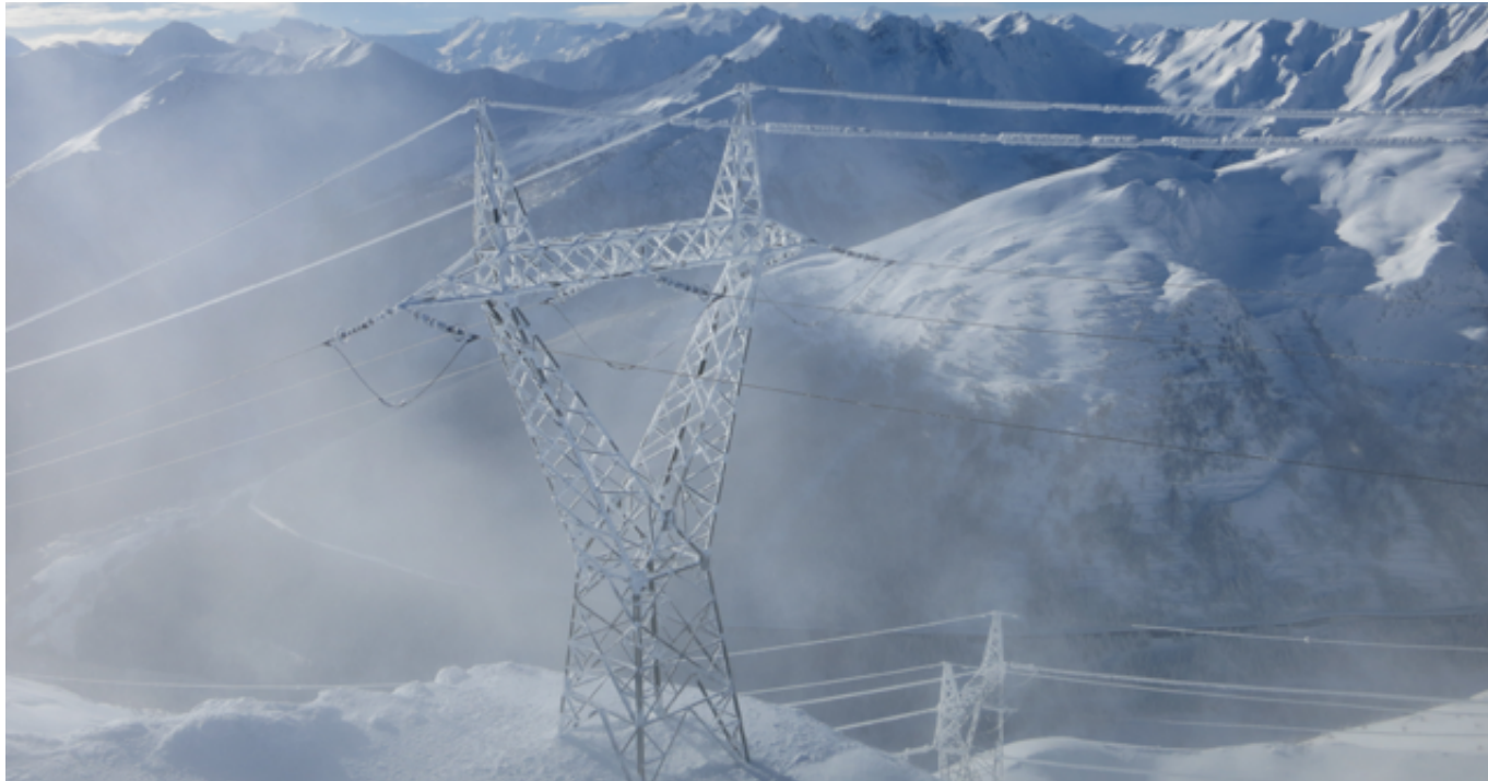
Snow-covered extra-high voltage power line
